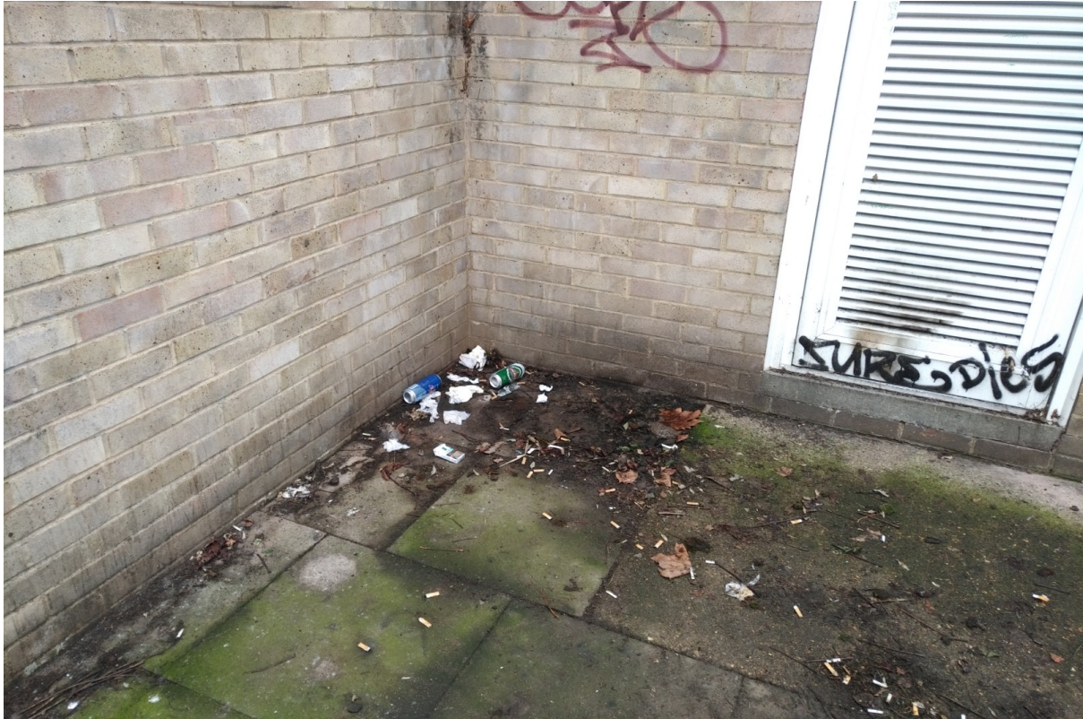
Photo 1 - Evidence of urination and alcohol related litter at South Grove Community Centre.
